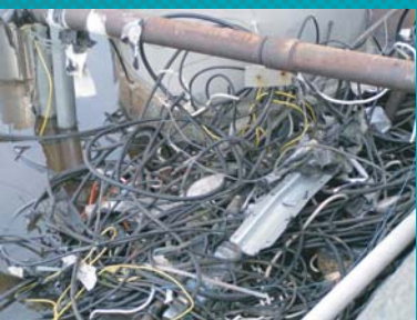
Damage caused by rooftop transmitter installation
