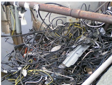
Damage caused by rooftop transmitter installation
