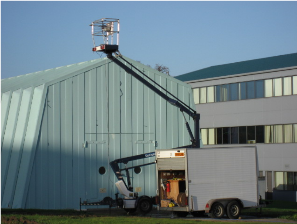
Figure 6: Picture of TV antenna mounted on a cherry pick
