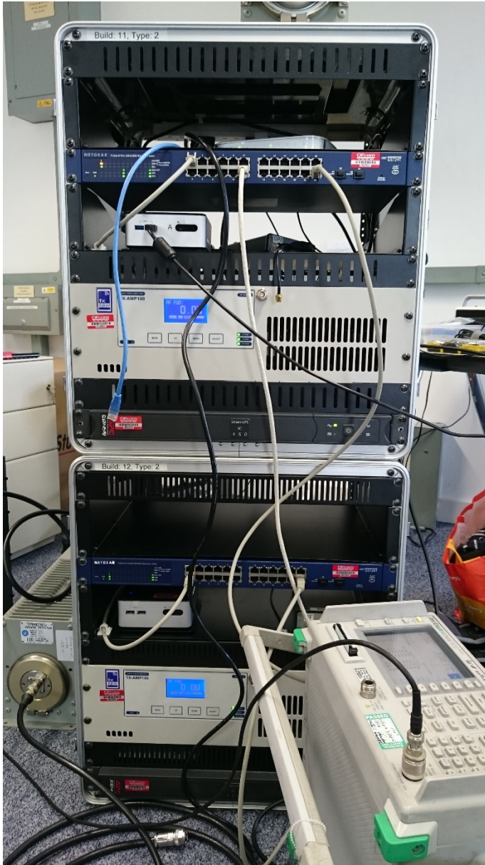
Figure A2: two of the 12RU trial racks undergoing functional testing
