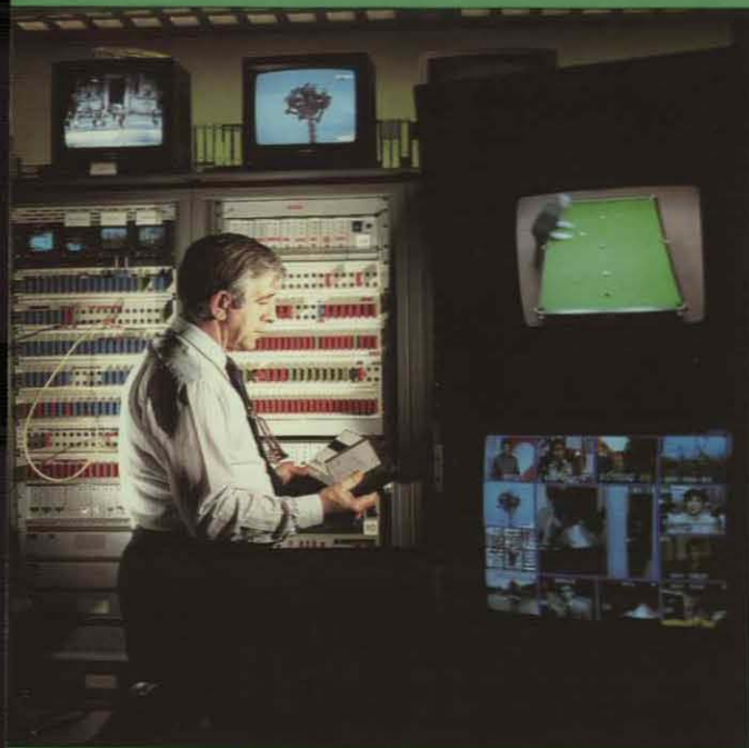
The control room at Westminster Cable
