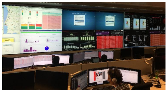
Typical utility distribution control room
